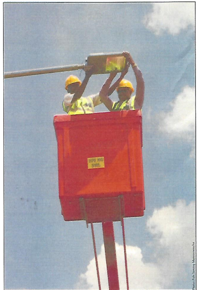
Nala Mayor CLLR Mogoje and Contract Worker Serame Mofokeng install LED lights
